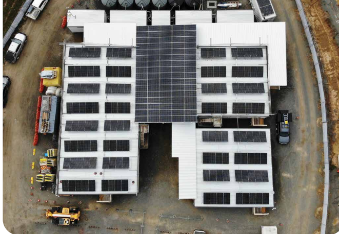
Princes Highway East Kilmany Solar, Victoria.
